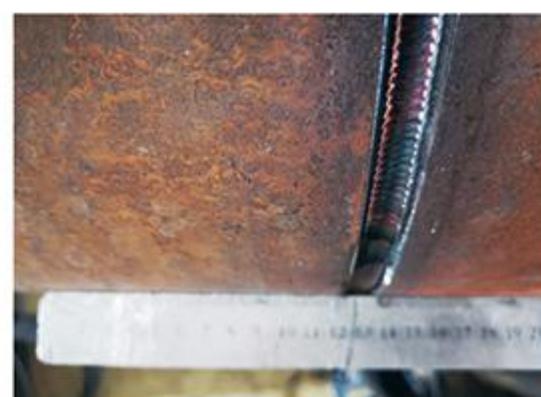
碳钢筒体手工氩弧焊焊接 Manual argon arc welding of carbon steel cylinder
