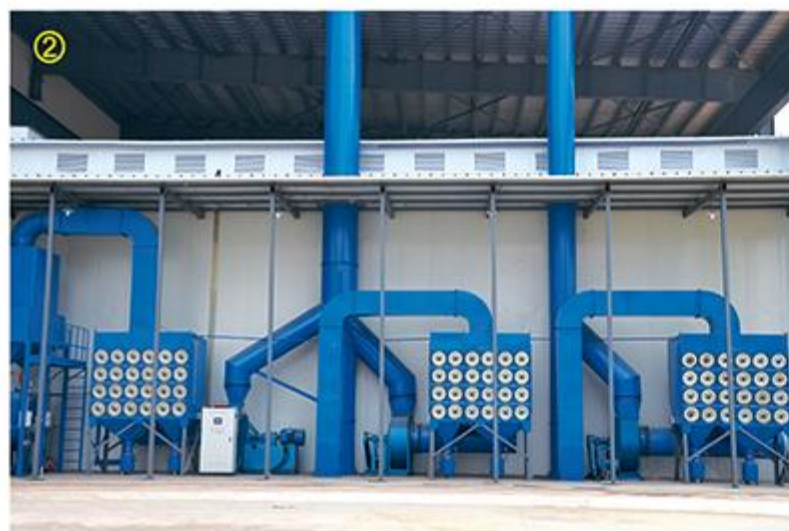
喷砂房 Sandblasting Room
