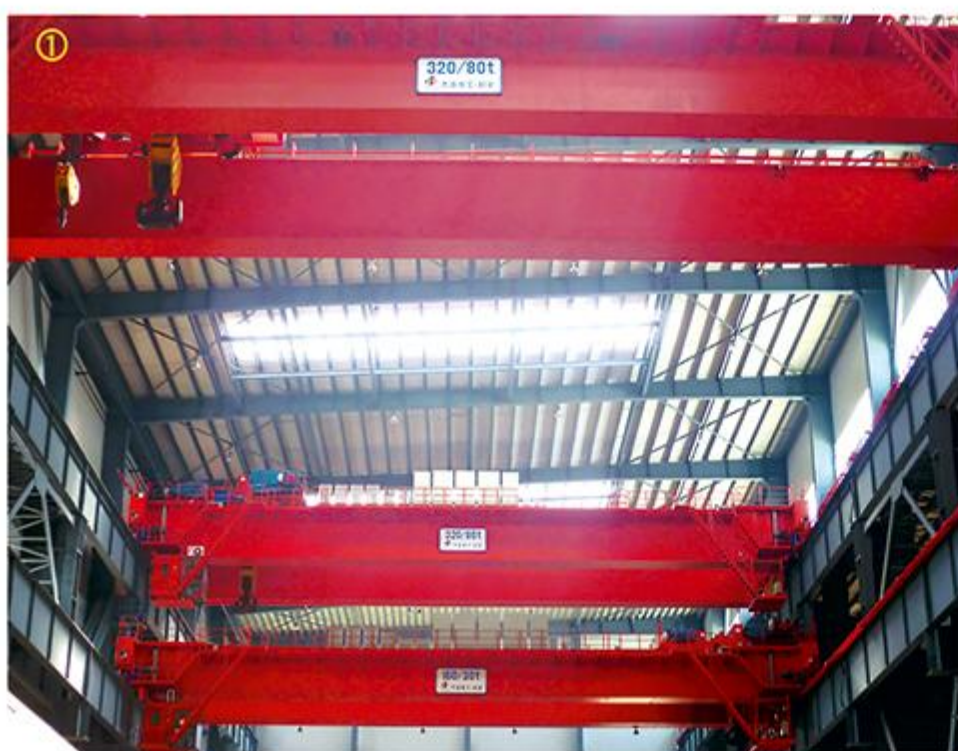
吊钩桥式起重机 Overhead Crane Hook
